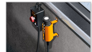
Pit connection box with E-Stop
